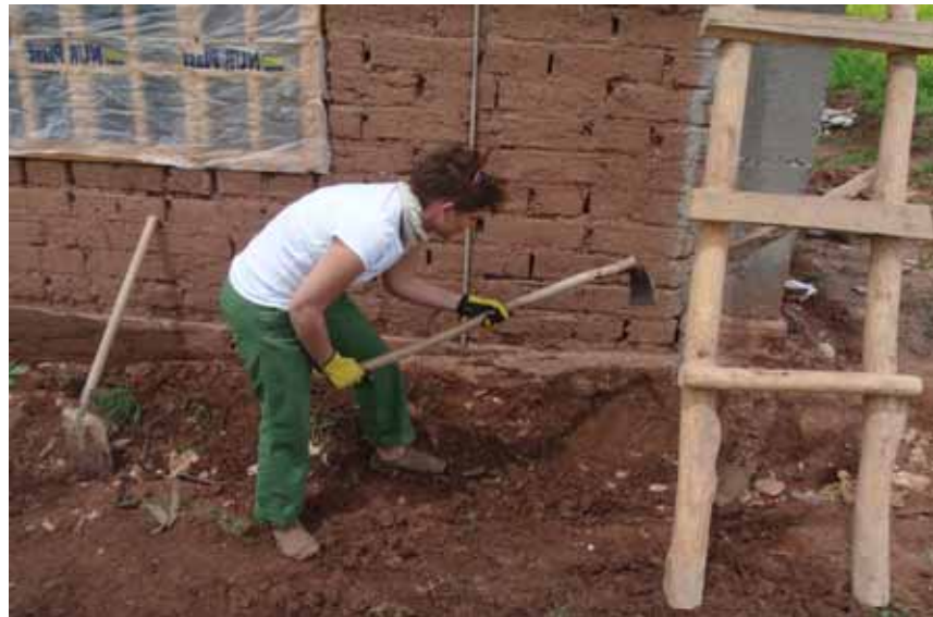
Melanie works on the hard ground getting ready for plastering of the walls at the home build in Tajikistan.
